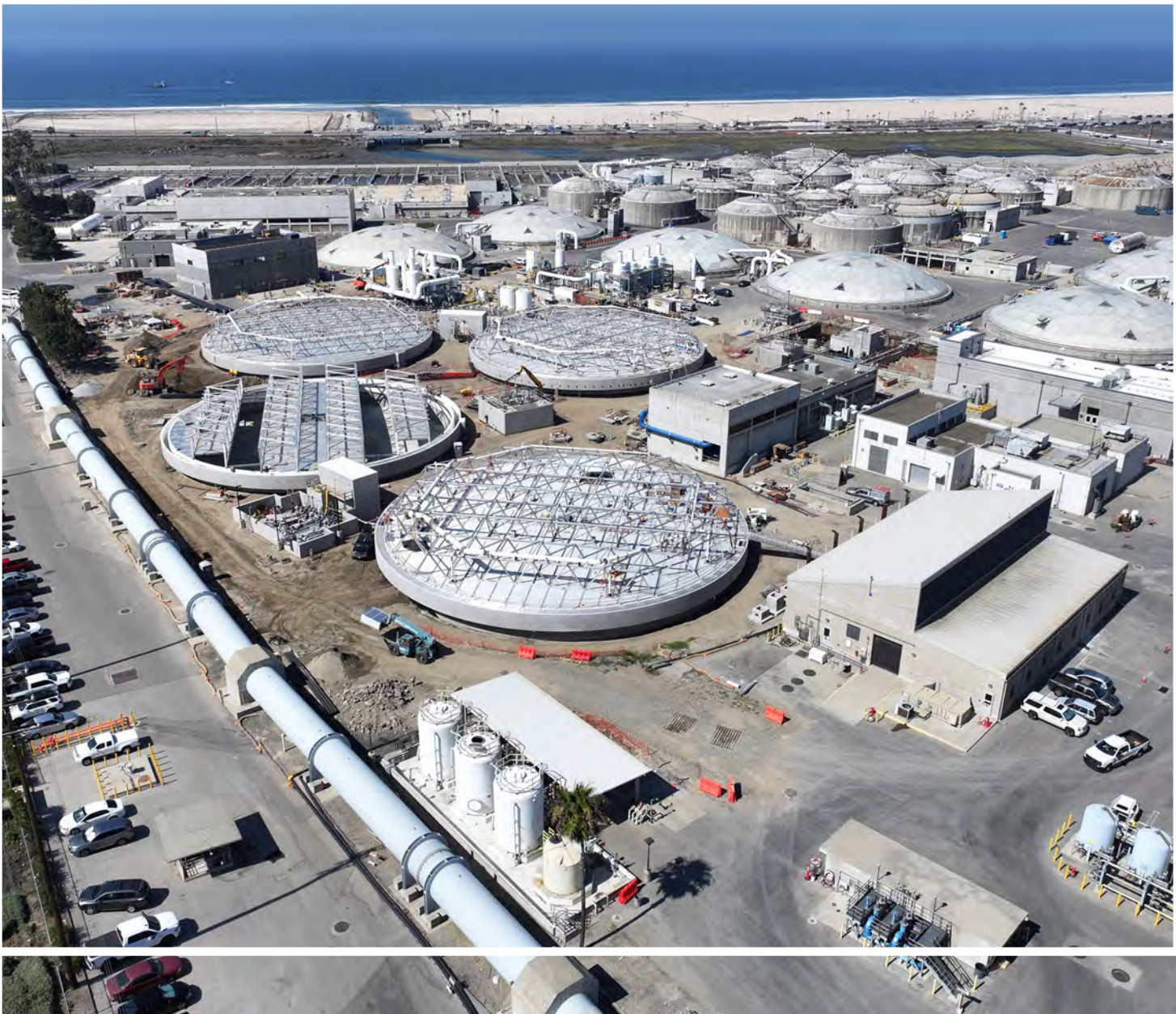
Four new primary clarifiers with truss-supported aluminum flat covers
