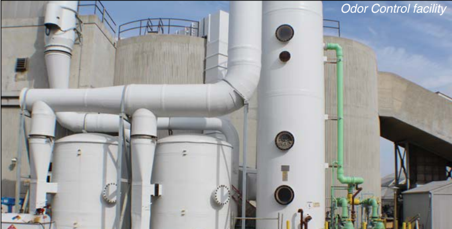
Odor Control facility
