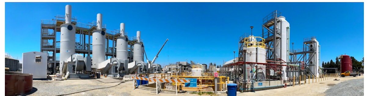
(TOP) The entire headworks area at Plant No. 1 is undergoing construction while keeping the existing facilities in service.
