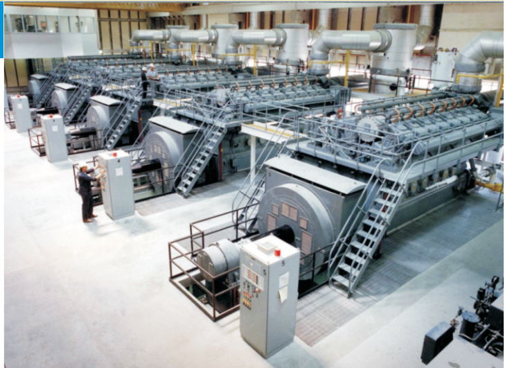
Central power generation system at Plant No. 2.
