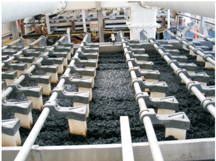
Excess water is removed before the biosolids are trucked away for reuse.
