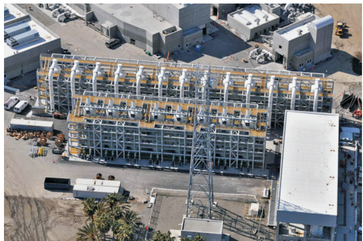
New air scrubber complex at Plant No. 2 costs about $255 million.
