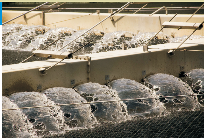
Trickling filters at Plant No. 1.
