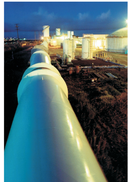
Ocean outfall pipe at Plant No. 2.
