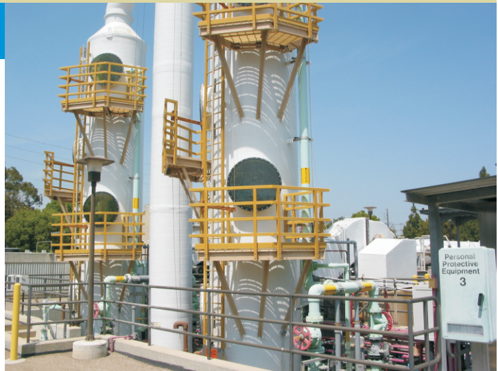
Odor control systems deodorize foul smelling air collected in the treatment plants.
