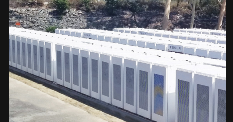
Tesla lithium battery storage system at Plant No. 1 in Fountain Valley.
