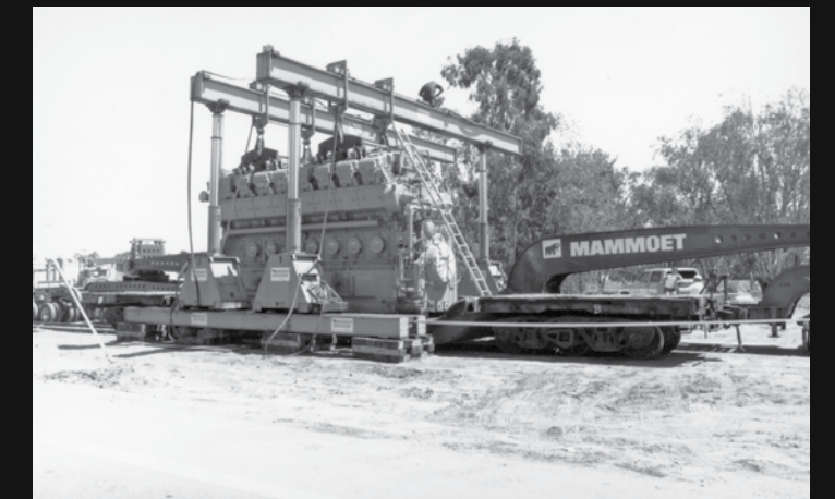
Installation of central generation engines at Plant No. 1.
