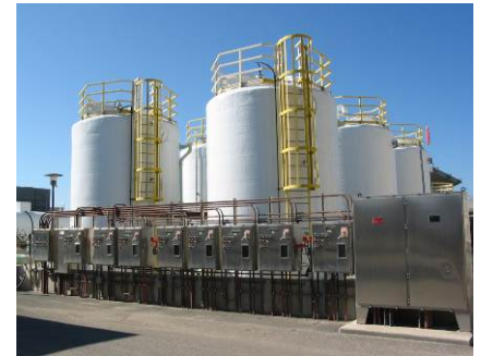
Disinfection chemical tanks at Plant No. 2.
