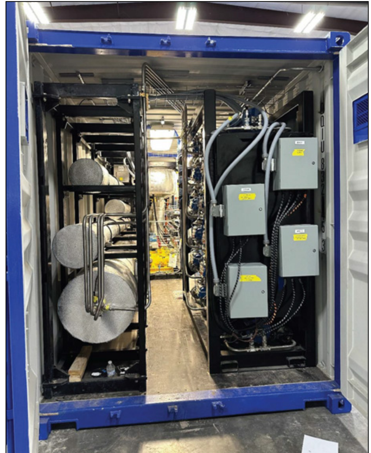
Heat exchanger skid and slurry pump skid fully installed into AirSCWO system.
