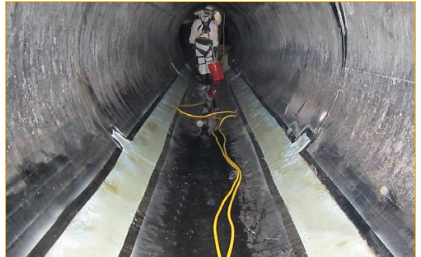
Crews working inside the pipeline on the Sunflower and Red Hill Interceptor Repair Project.
