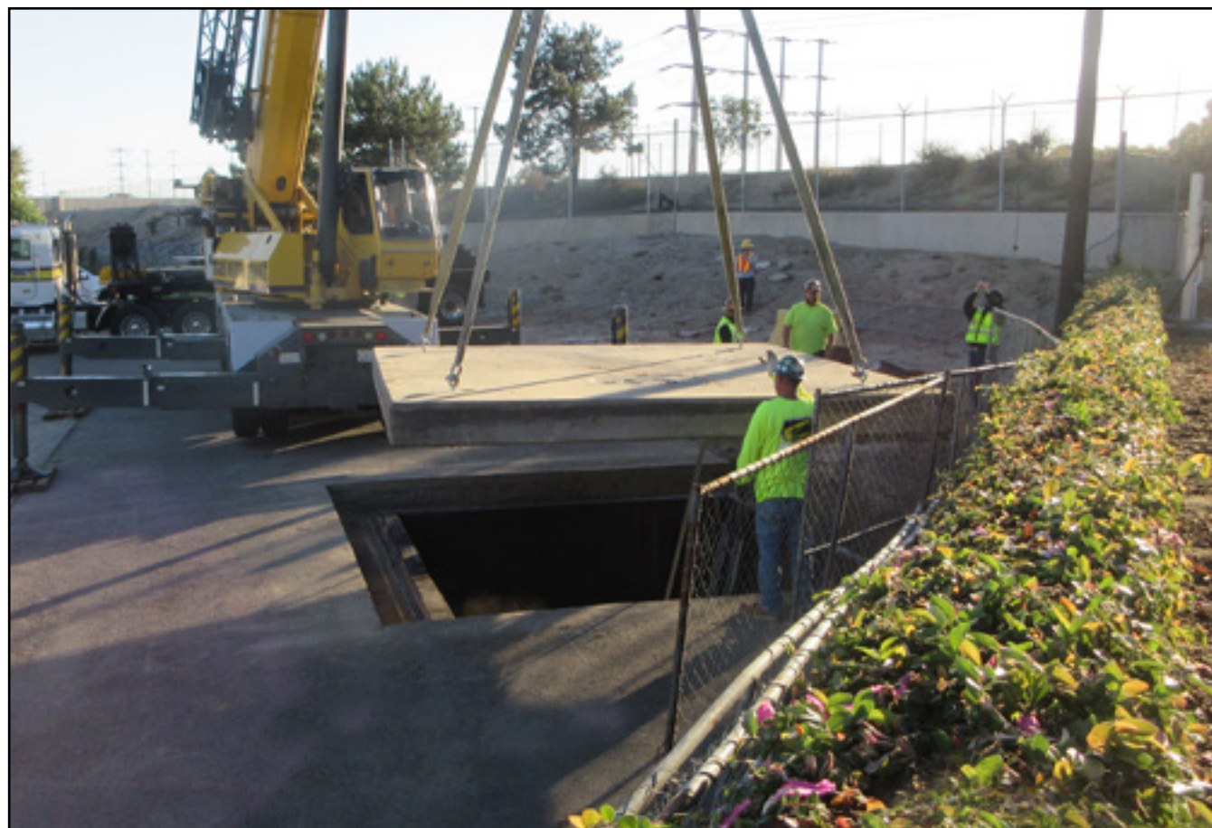
Removing manhole cover on the Santa Ana Trunk Rehabilitation at Plant No. 1 Project.
