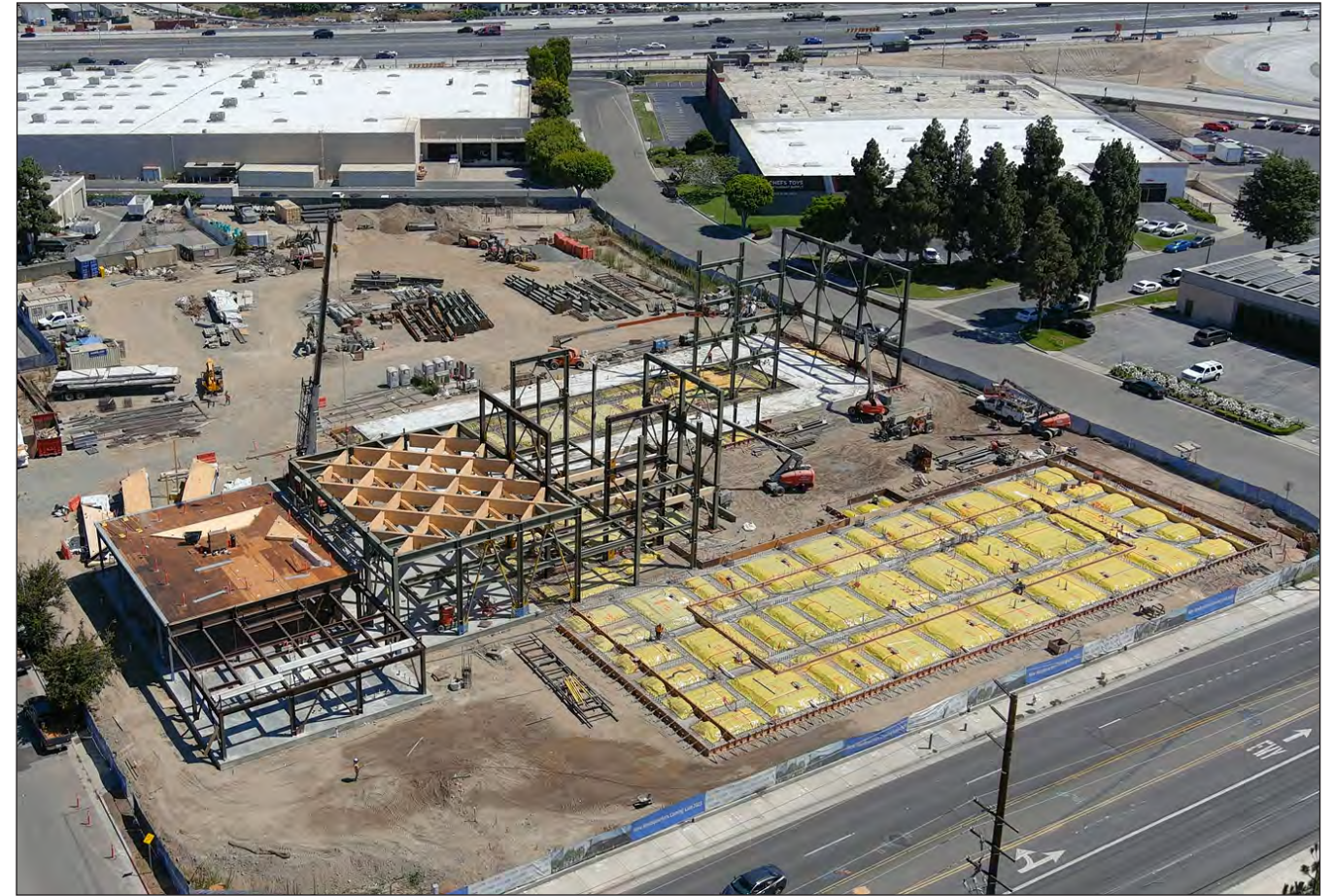
The foundation work is completed and vertical structural steel elements and mass timber are starting to go up on the Headquarters Complex Project.
