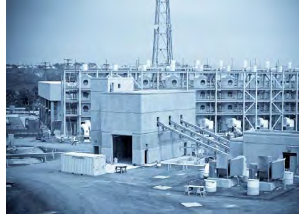
New odor control facilities in construction at Treatment Plant No. 2 in Huntington Beach.
