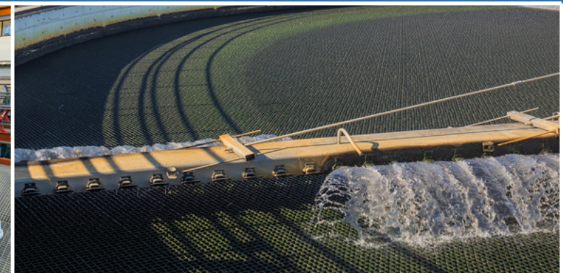
Left to right: Centrifuge; trickling filter at Plant No. 1 in Fountain Valley.
