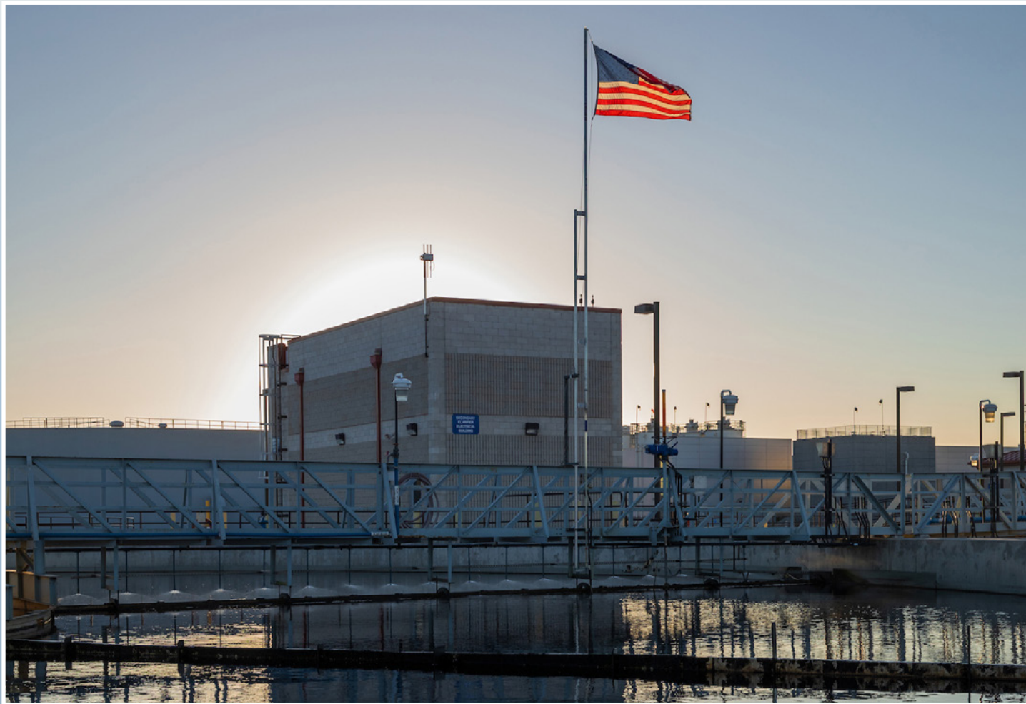
Secondary clarifier at Plant No. 1 in Fountain Valley.
